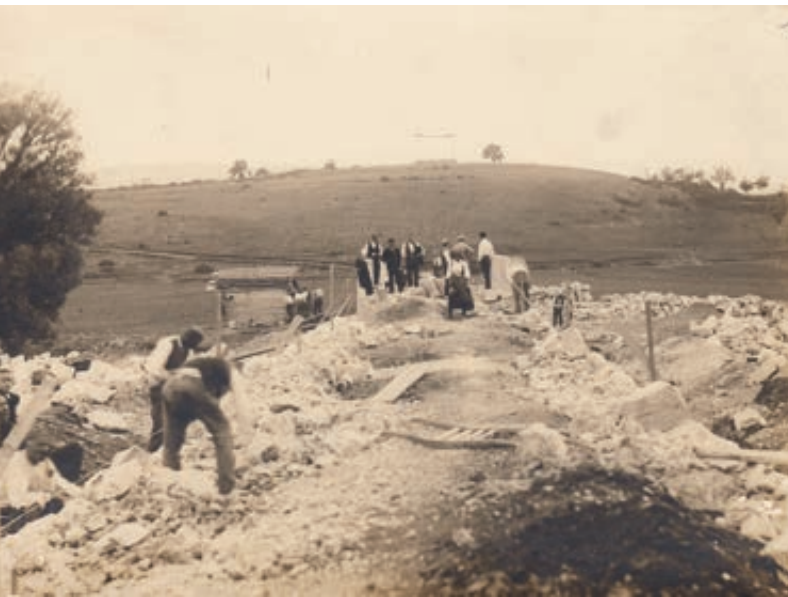
Fig. 9. Construction of the access road and the bridge at the foot of Paraćeva Glavica, 1929 (Marin Maraso- vić Archive, inv. no. AFMM-10.4).
